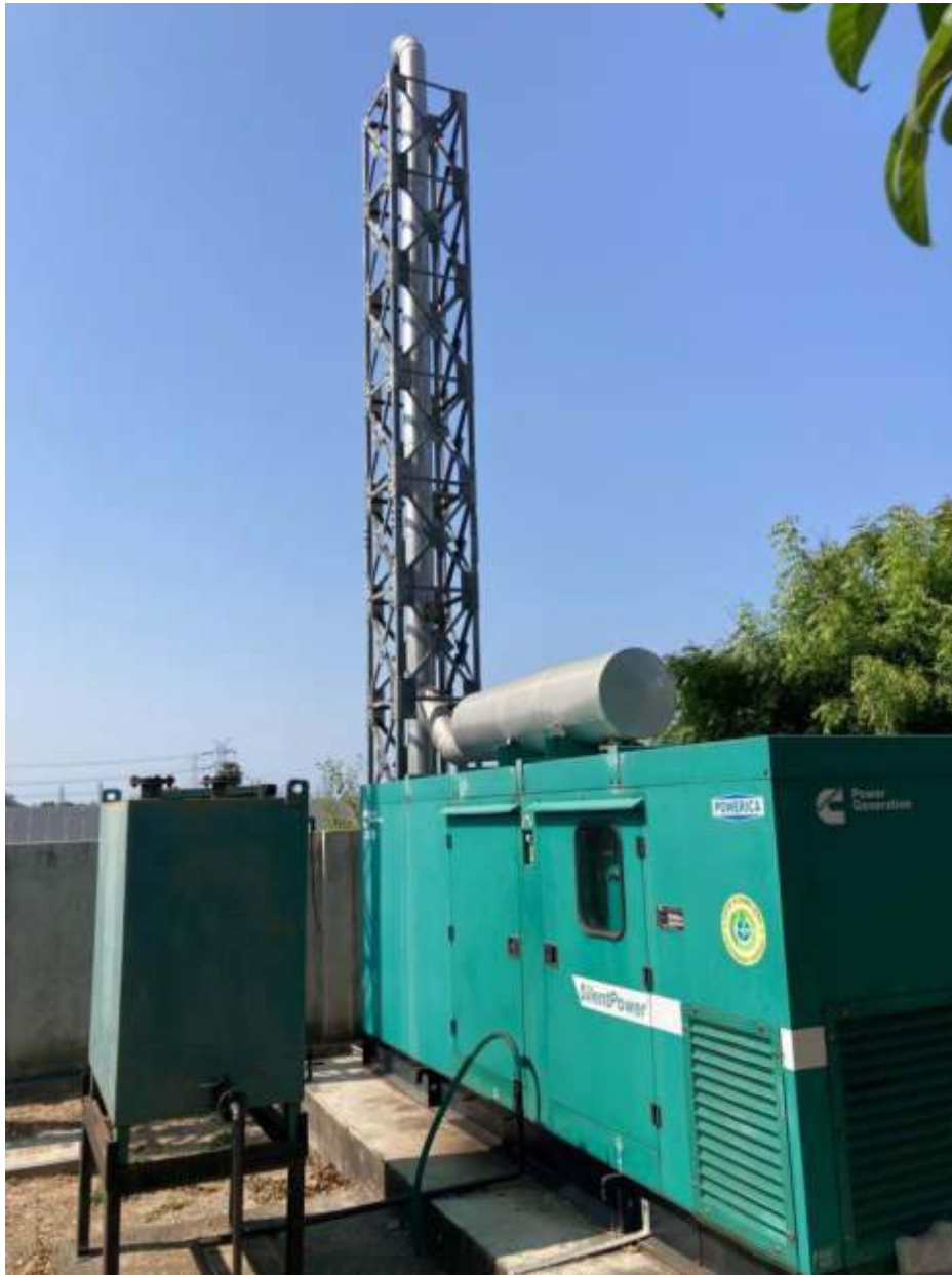
Dg set at Tower A1 – 320 KVA
