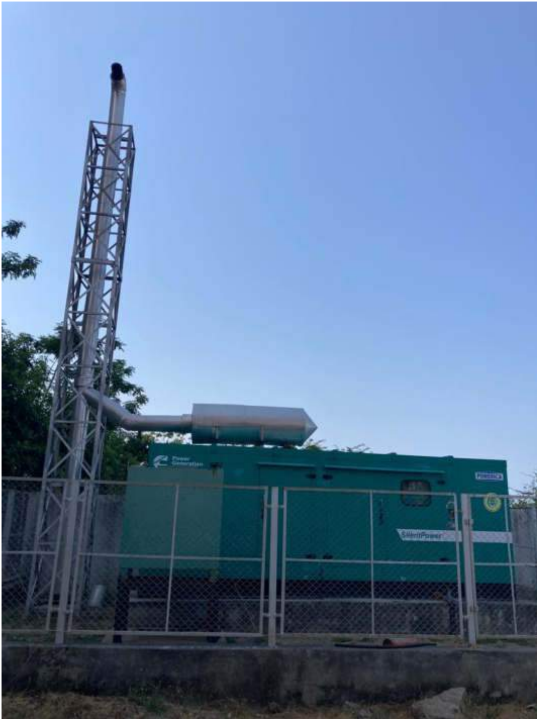
Dg set at Tower C1 – 500 KVA
