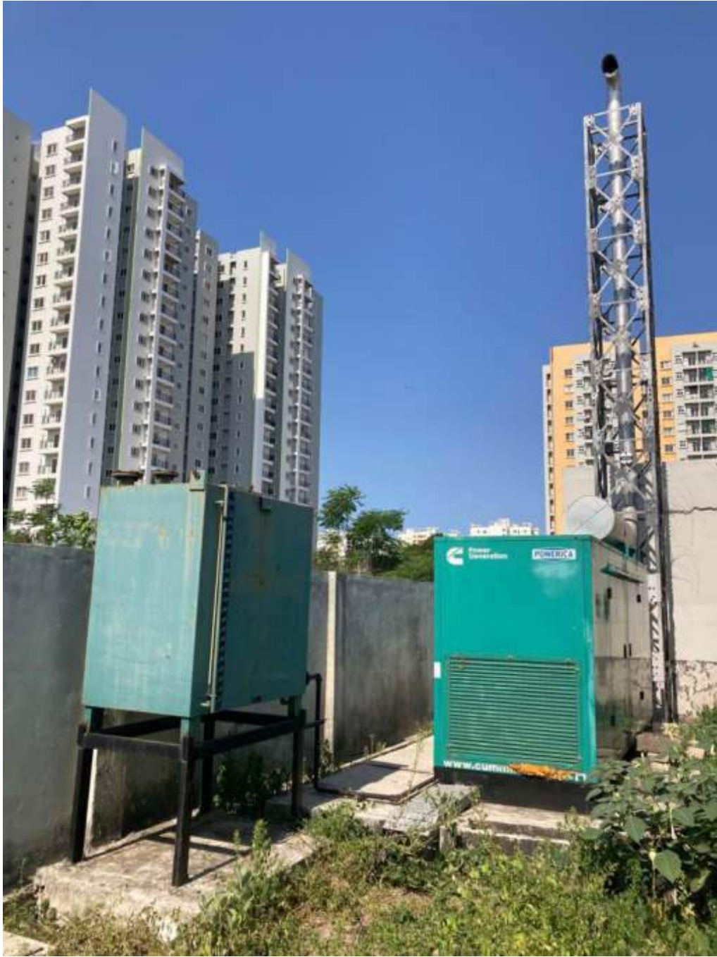
Dg set at STP – 160 KVA
