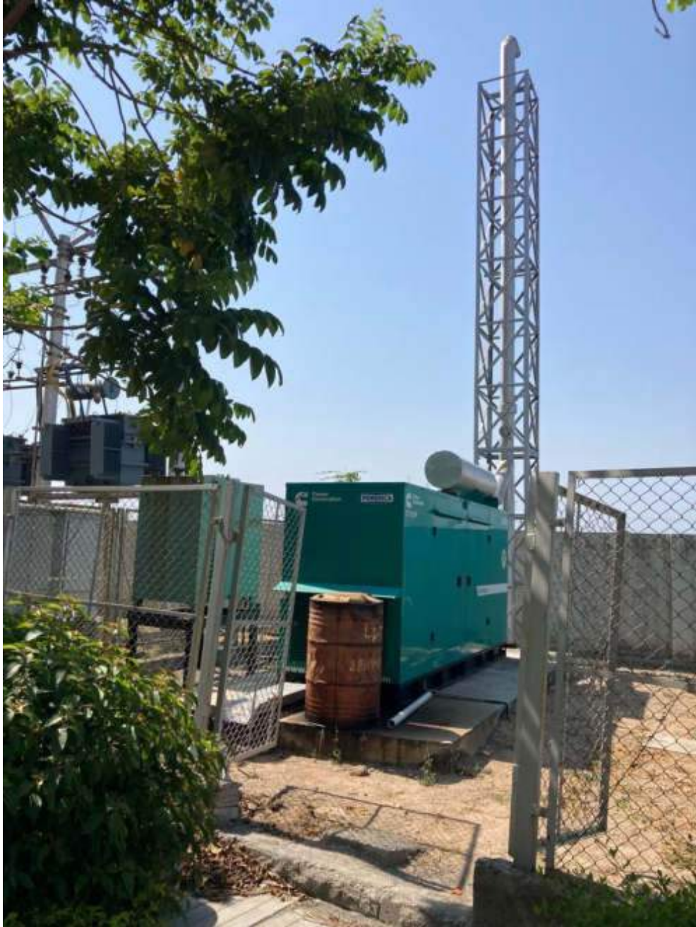
Dg set at Tower A1 – 125 KVA
