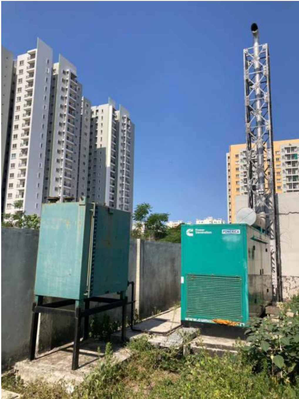
DG set at STP – 160 KVA
