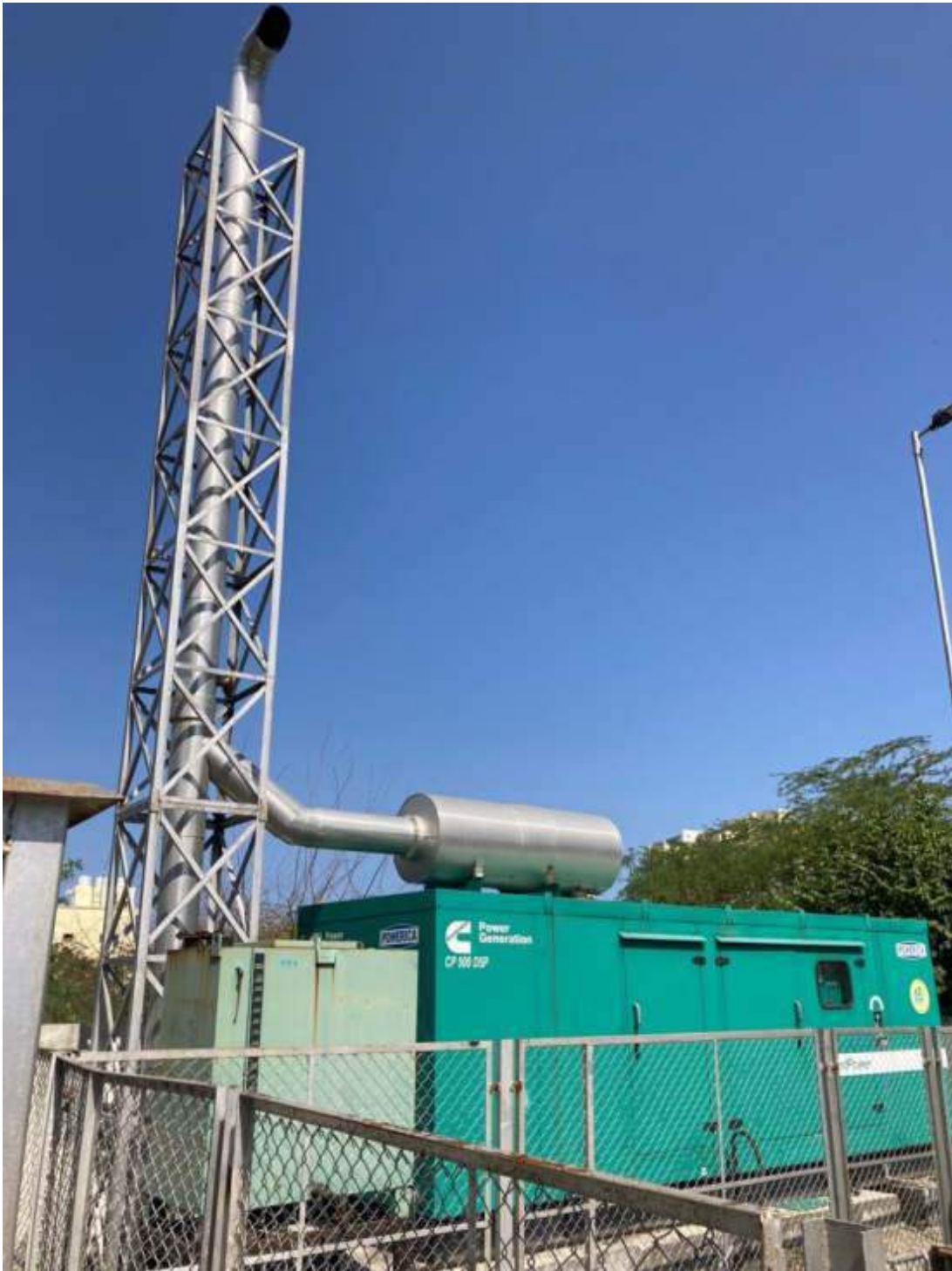
Dg set at Tower C7 – 500 KVA
