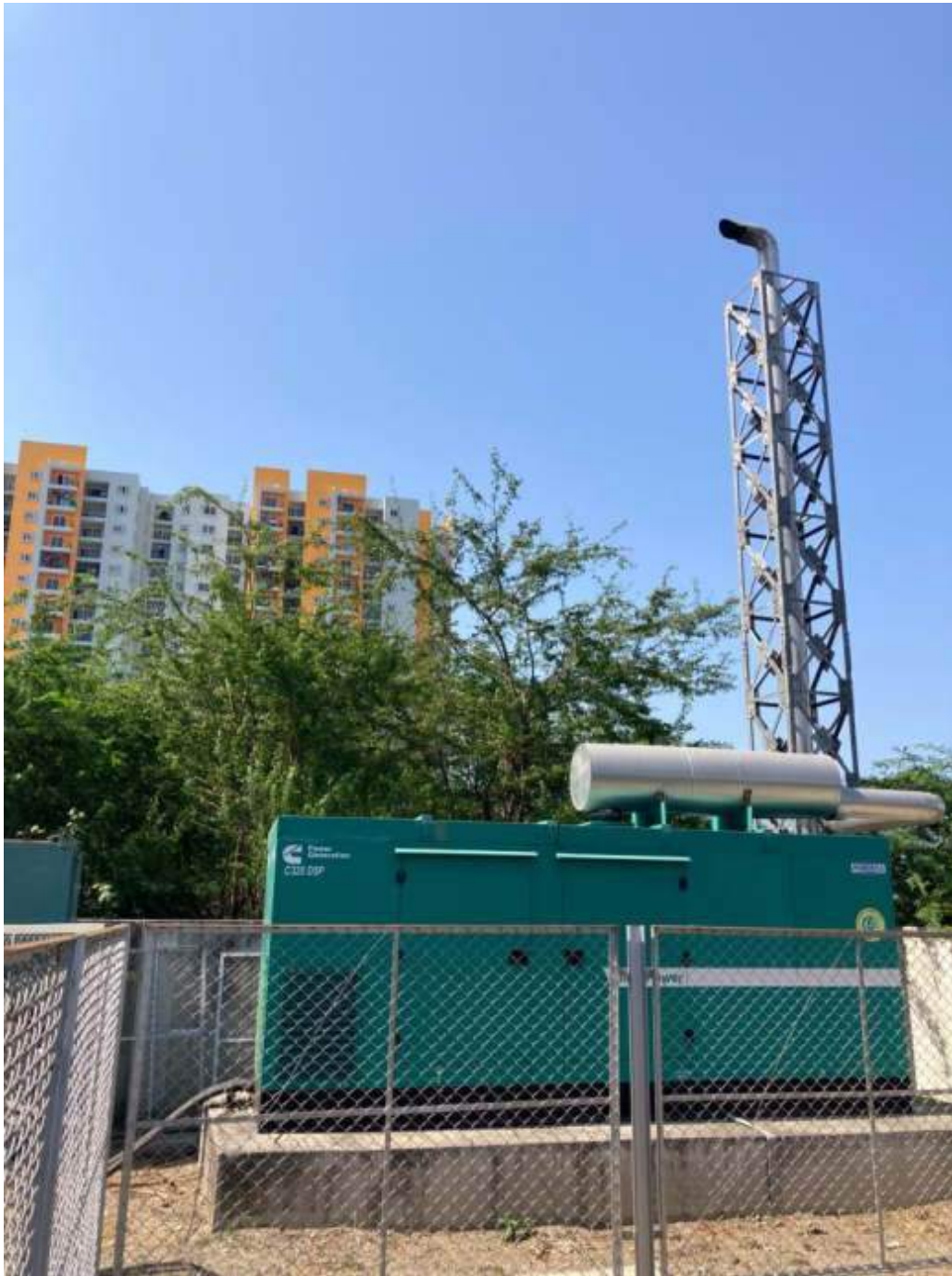
Dg set at Tower B1 – 320 KVA
