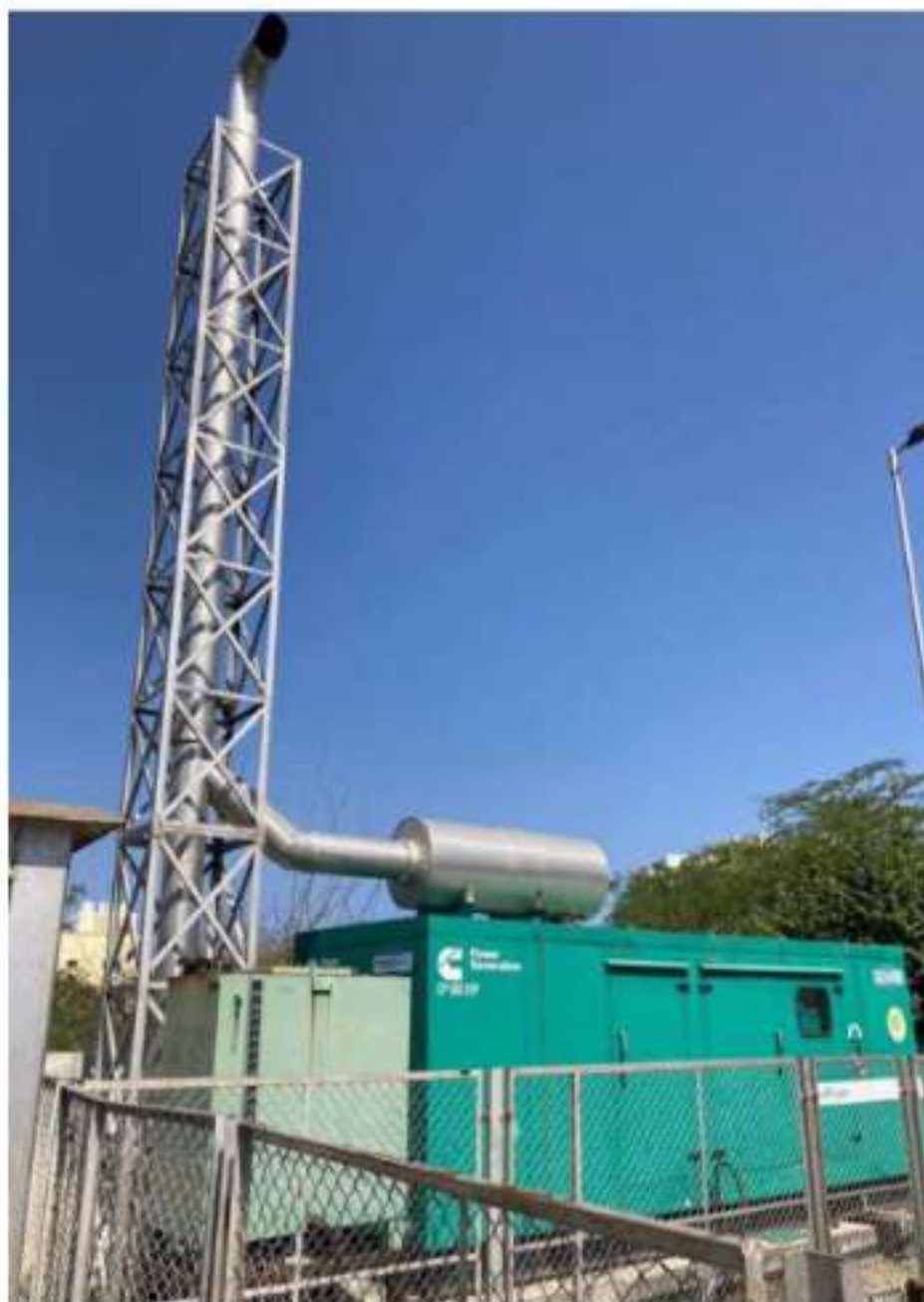
Dg set at Tower C7 – 500 KVA
