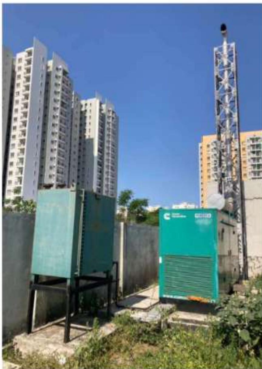
DG set at STP – 160 KVA
