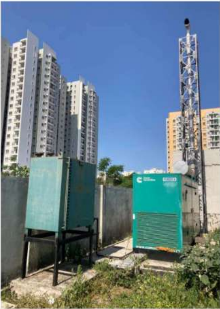
Dg set at STP – 160 KVA
