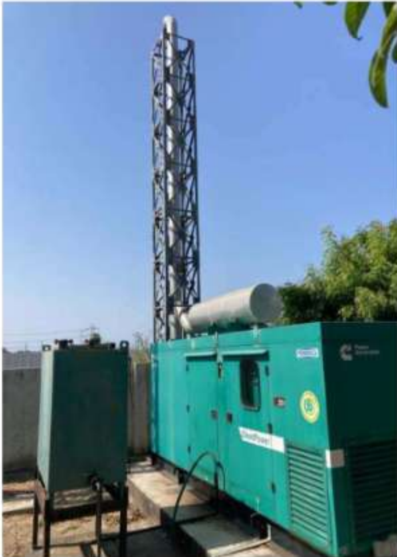
Dg set at Tower A1 – 320 KVA
