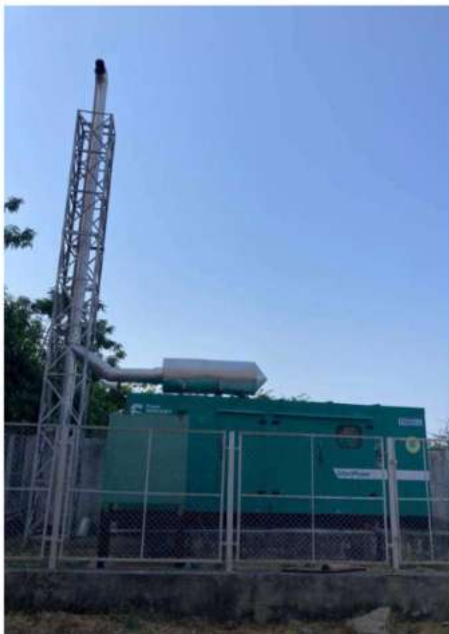
Dg set at Tower C1 – 500 KVA
