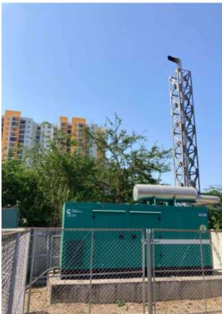
Dg set at Tower B1 – 320 KVA
