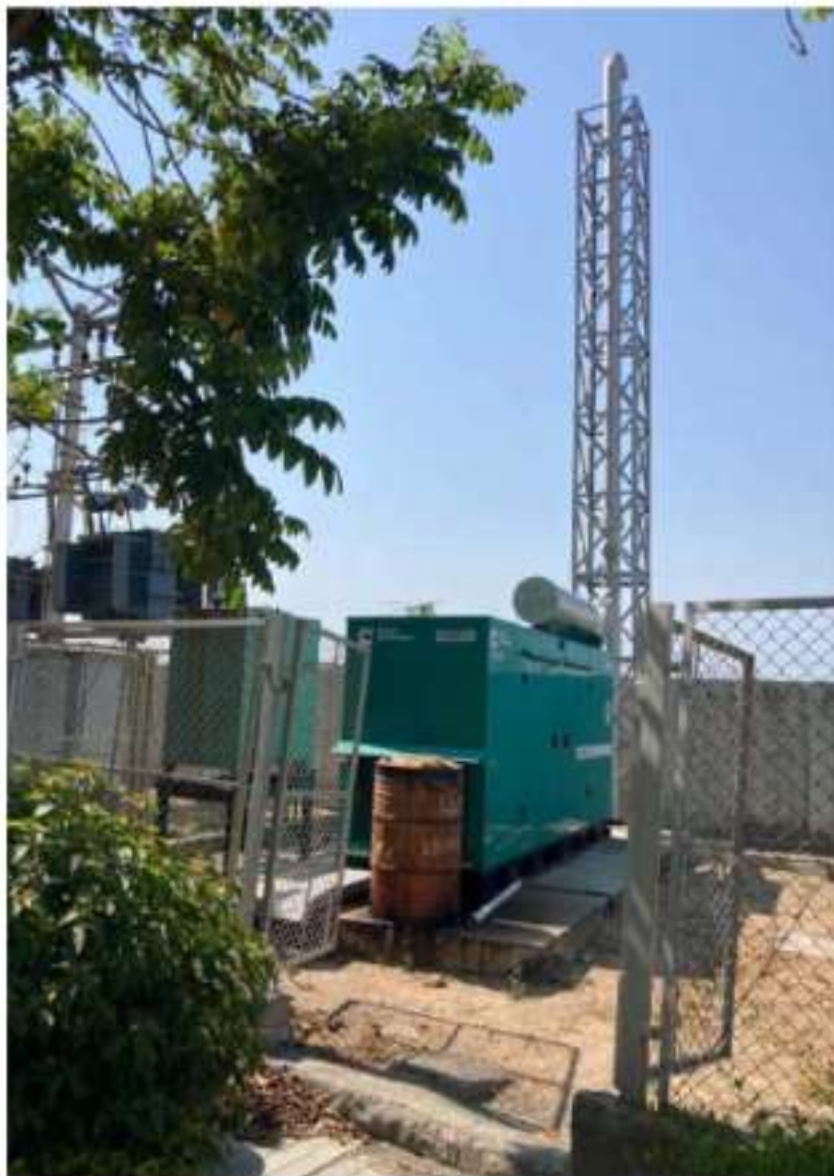
Dg set at Tower A1 – 125 KVA
